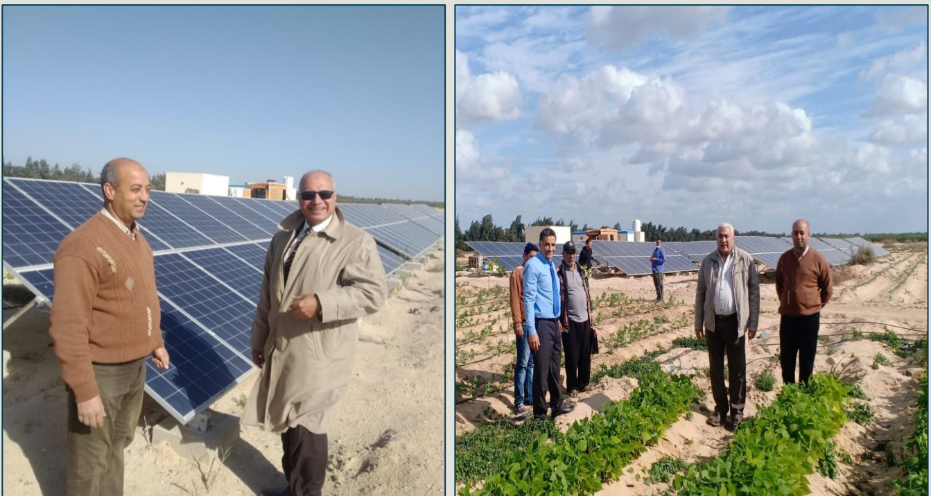
Figure 5-2 installed solar panels
